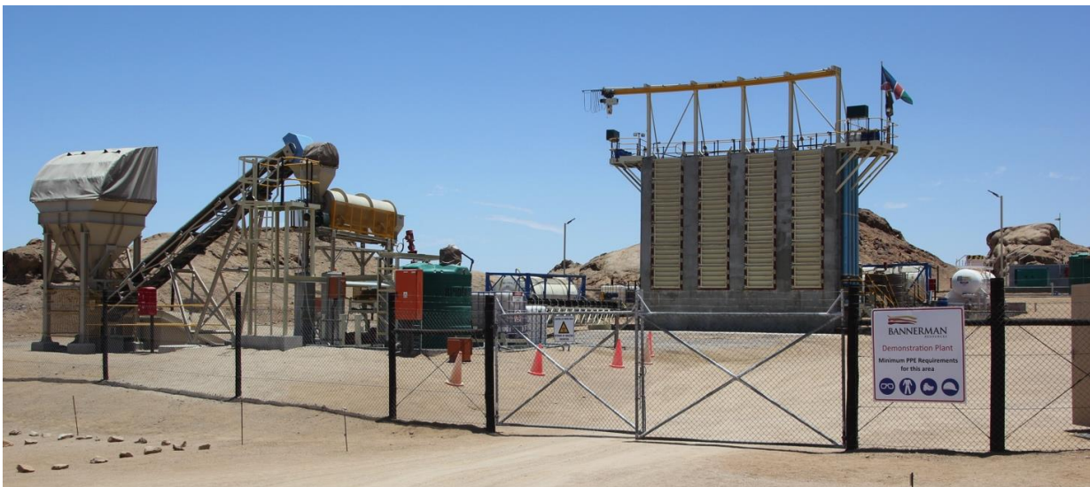
Figure 1 - Etango Heap Leach Demonstration Plant
