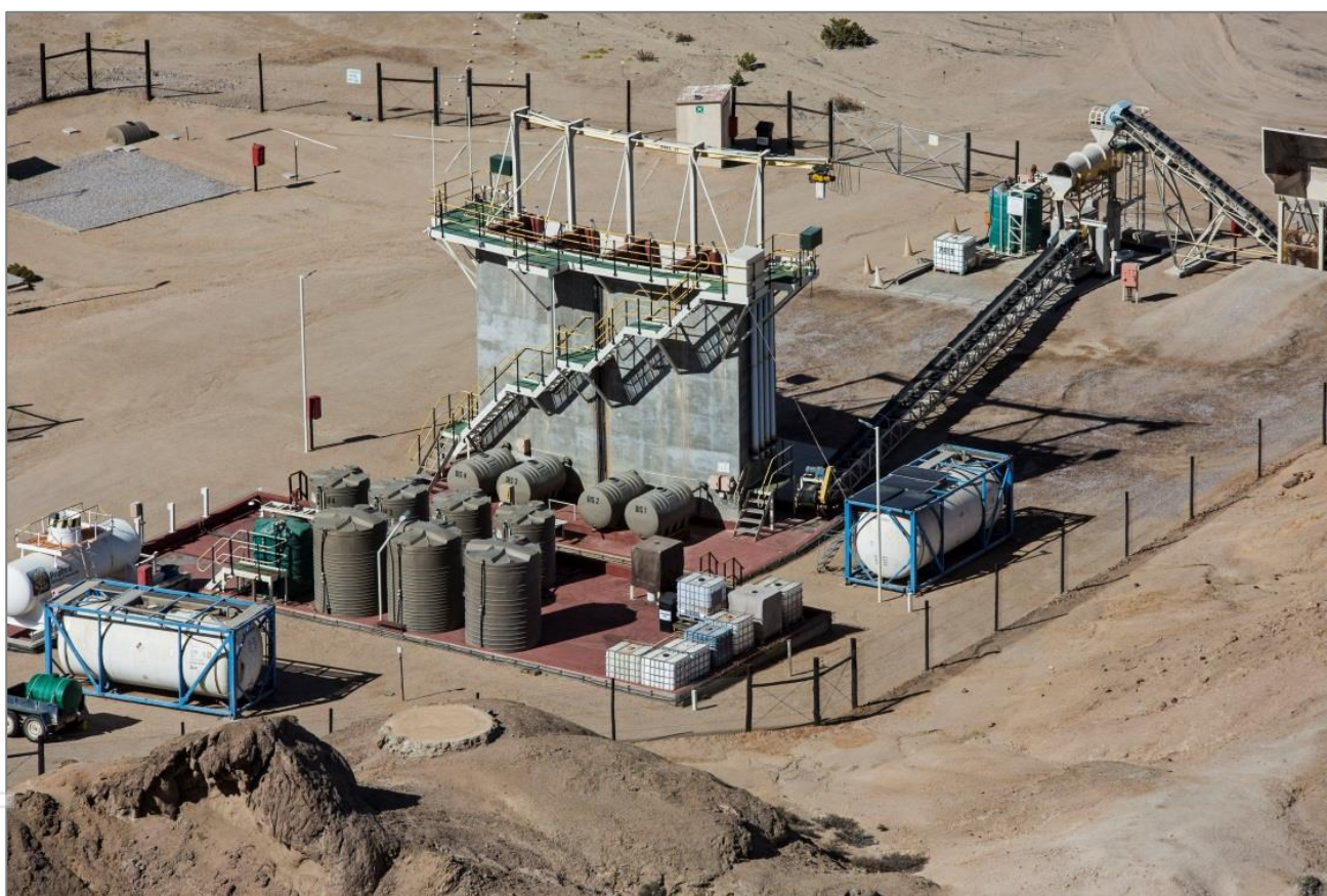
Figure 1: The Etango Heap Leach Demonstration Plant has comprehensively de-risked the acid heap leach processing route
